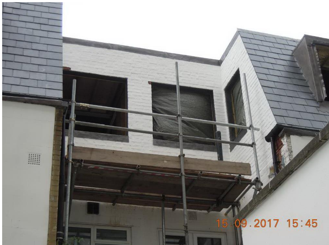
Front elevation of Nos. 110-126 Westbourne Terrace Mews (top) and sheer second floor window openings to Nos.118 and 120 Westbourne Terrace Mews (bottom).
